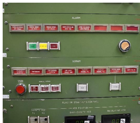
One of the control panels of UTR
